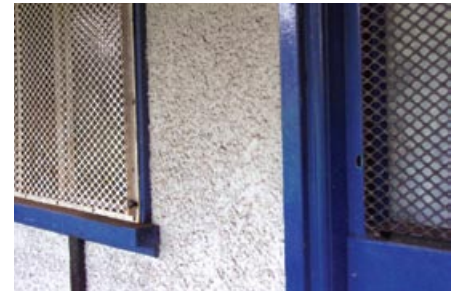
Figure 33 Chrysotile pebble-dash exterior wall coating
