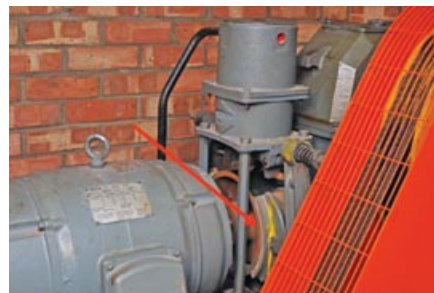
Figure 42 Asbestos brake lining on output shaft of AC motor
