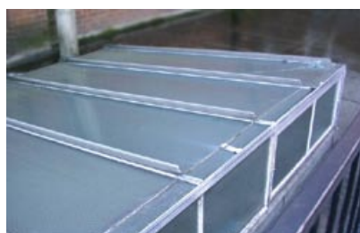
Figure 31 Chrysotile string on skylights
