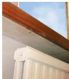
Figure 20 AIB panel between radiator and window
