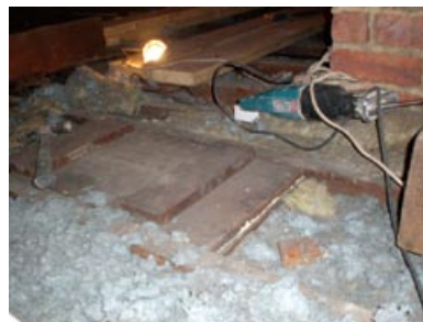
Figure 6 Loose asbestos used as loft insulation
