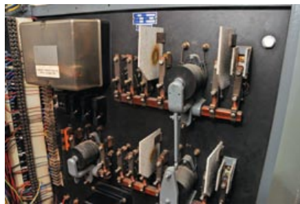
Figure 50 Open electrical switchboard with asbestos flash guards
