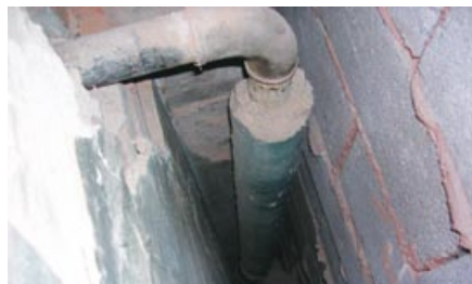
Figure 9 Lagged pipe in wall cavity
