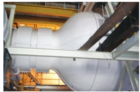
Figure 51 Vessel clad in amosite insulation
