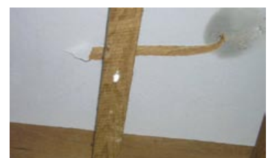
Figure 25 Chrysotile paper on strawboard ceiling panels
