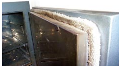
Figure 26 Asbestos rope seal on drying oven
