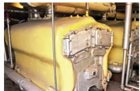
Figure 13 Amosite lagged boiler with hard plastic coating
