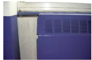
Figure 19 AIB behind school radiator unit
