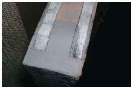
Figure 14 Asbestos panels inside fire door
