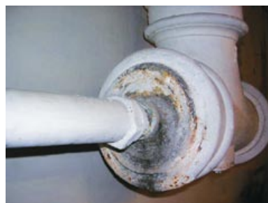
Figure 30 Amosite and chrysotile packing on waste pipes
