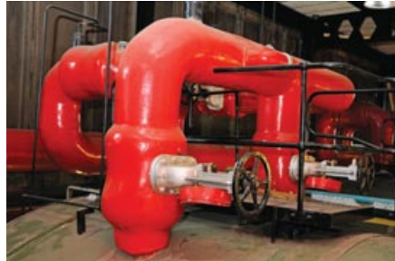
Figure 48 Asbestos-insulated supply pipes
