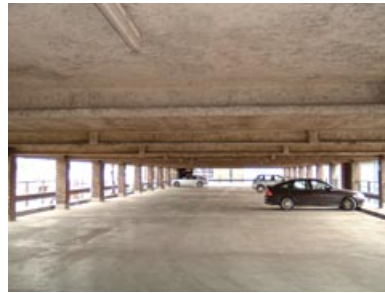
Figure 7 Sprayed limpet on car park roof
