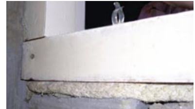
Figure 27 Amosite asbestos rope packing on riser door frame
