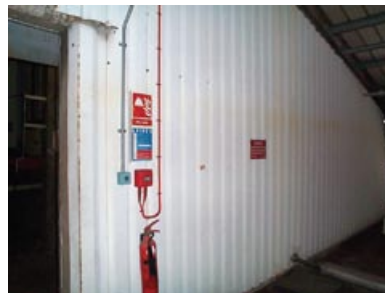
Figure 38 Chrysotile/bitumen coating under metal cladding
